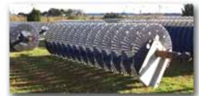
Replaced Disc Rotors
